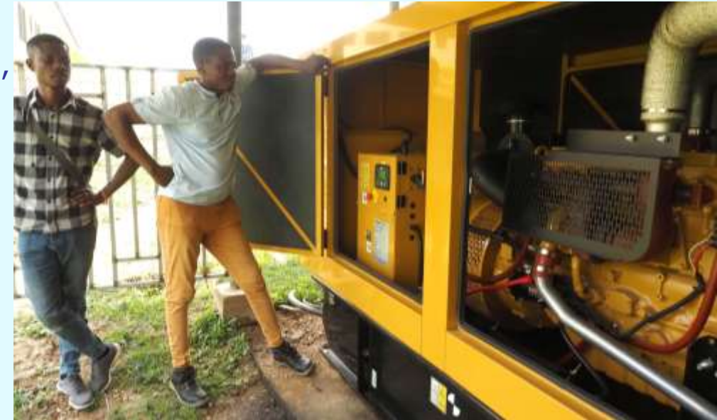
Diesel generator Maria Theresa Hospital, Dodi Papase, Ghana, 2026
